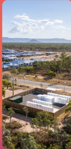
Battery Energy Storage
