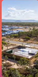
Battery Energy Storage
